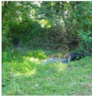
Basin at DCCD Tour Site #7
